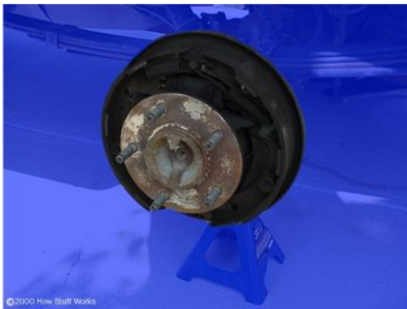
Figure 3. Drum brake without drum in place
